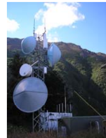
The ALMR Asset Manager completed inventory of Air Force and Army assets at 50 locations this summer, including this site at Hope.
